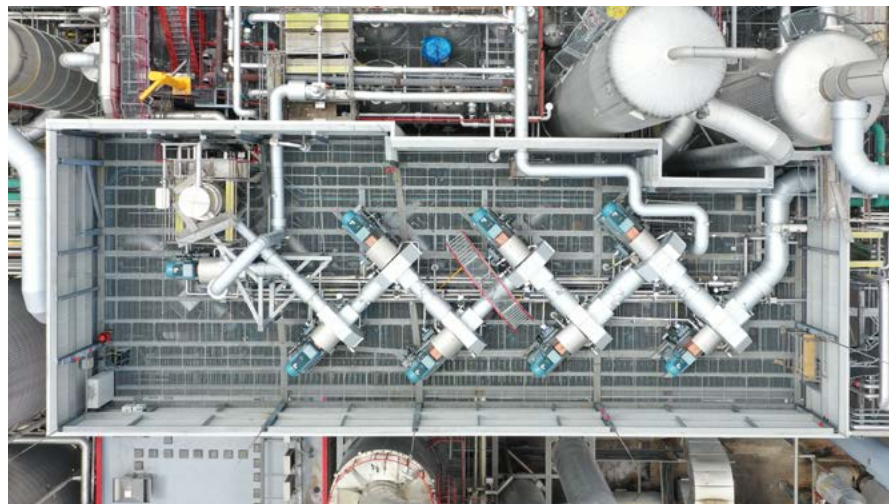
Heat pump technology: Vapor compression line with PILLER MVR Blowers
